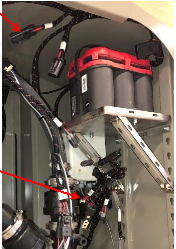
Step 1 Pump Stop
