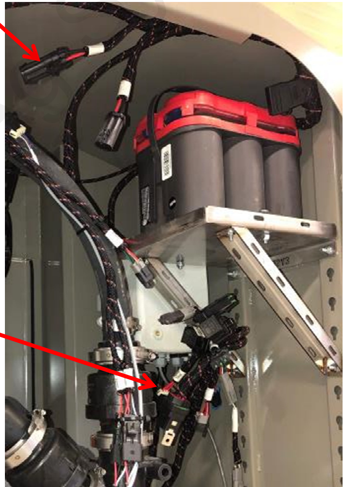
Step 1 Pump Stop
